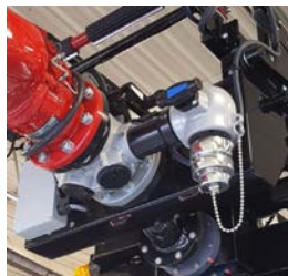
Figure 4-16. Aerial Standpipe Connection
