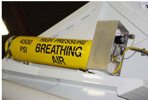
Figure 3-20. Breathing air system high-pressure cylinder
