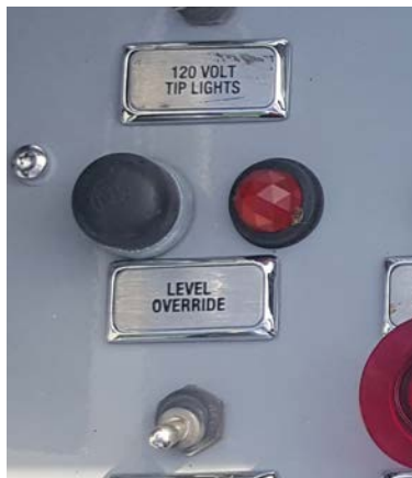
Figure 4-20. Level Override Control
